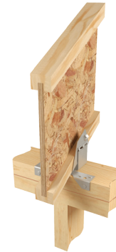
Typical TMP installation
